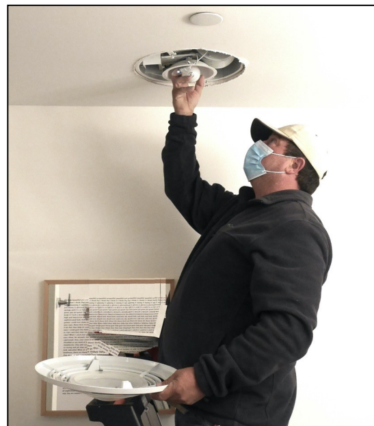
Replacing lights is part of Justin Routier's normal work day.
